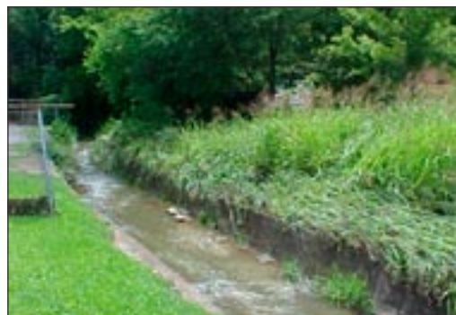
Recently Flooded Ditch
